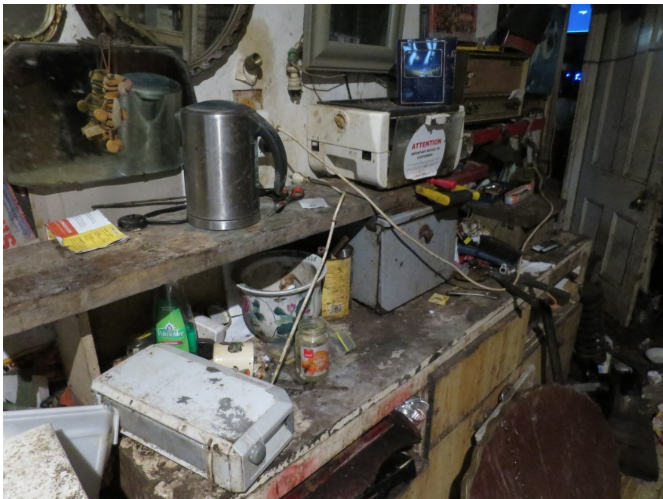
Photograph of kitchen illustrating severe domestic squalor.
